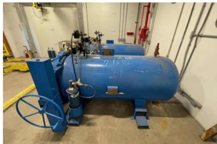
Proactive, special secondary containment vessels for chlorine gas cylinders have provided readily accomplished safety enhancement for employees, as well as the public.
