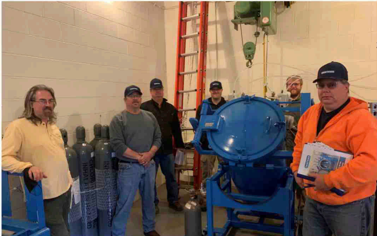
The installation of the special secondary containment vessel for chlorine gas cylinders at the Ludington, MI, WWTP was the first use of the innovative technology in that state. From left to right are Kyle Bond, Water Circuit Rider for the Michigan Rural Water Association; Plant Operator John Dickinson; Plant Operator Jared Beyer; Plant Operator Kevin Taranko; Plant Superintendent Chris Cossette; and Plant Operator Gary Walton.
