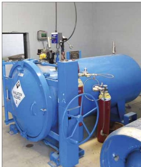
Two one-ton ChlorTainer secondary containment vessels for chlorine gas cylinders were installed, in the room originally designed for the bleach tanks and associated equipment, to help allow for safe delivery of 160 ppd of chlorine for pre-and post-injection feeds, as well as helping for safe changeout of spent cylinders. The compact installation left plenty of room for a shop for trucks and backhoes, negating the need for a separate shop building.
