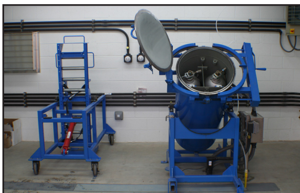
Booster station installations also use ChlorTainers designed for 150-lb. chlorine gas cylinders.
