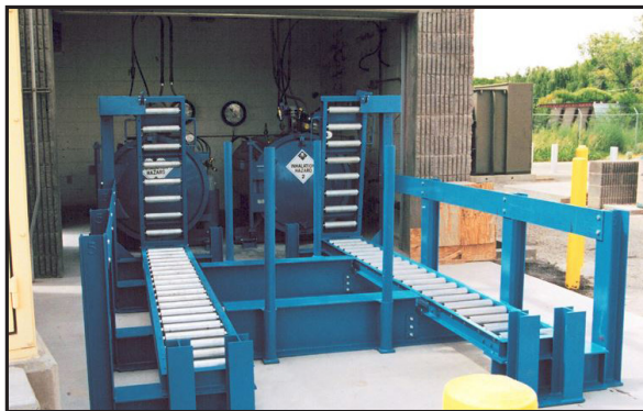
Booster station installations typically feature two 1-ton units, with drawbridge loading, side by side.
