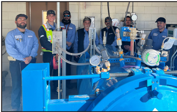
Special secondary containment vessels for chlorine gas cylinders have provided long-term, readily accomplished safety enhancement for employees, as well as the public, via installation at booster stations, as well as at two WWTP's and a WTP. The units are reported as requiring only simple, easy maintenance, and with operators easily trained for routine use.
