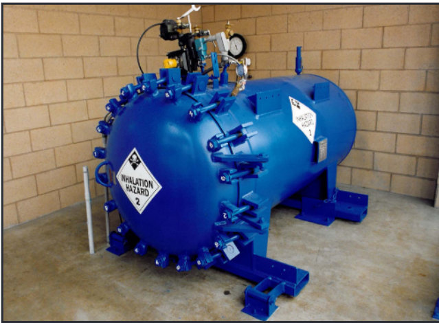
A refurbished, 1-Ton ChlorTainer secondary containment vessel with an 18-bolt door, like this one, was provided for an interim installation.
