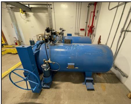
A failsafe valve ties into the chlorine leak detection sensor, so that in the event of an external release, a nitrogen and electric powered failsafe valve will close, stopping it completely. Any leak or release of chlorine gas from the vacuum line downstream of a vacuum regulator (mounted on top of vessels) will lose the vacuum condition, and cause the vacuum regulator to close, stopping the flow of chlorine gas to the vacuum line.
