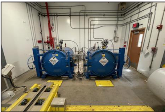
As an added assurance toward ease of use by plant operators, the utility's consulting engineers collaborated with the containment vessel manufacturer on an optional innovation of adding an electronically controlled sled, with a push-bar, to move the cylinders during changeout, instead of having operators physically pushing them. Operators had become disillusioned with previous installation placed in a room that was too small.
