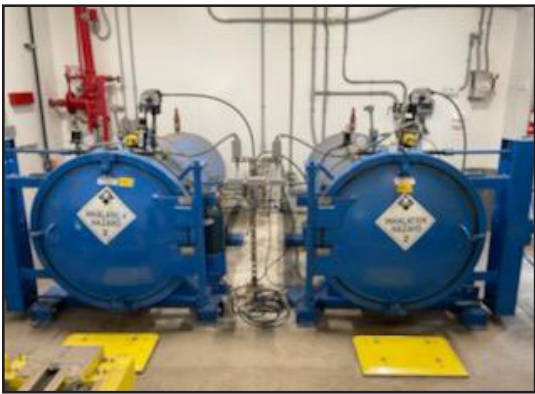
Secondary containment vessels for chlorine gas cylinders were installed as a reliable, lower-maintenance, enhanced leak safety alternative to wet and dry scrubber systems. The utility's consulting engineering firm had noted "significant savings in maintenance and insurance costs" by being able to "decommission a scrubber system and its associated appurtenances (at end of its useful life)," and not replacing it with a new scrubber.
