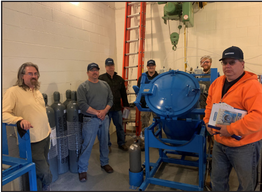
The installation of the special secondary containment vessel for chlorine gas cylinders at the Ludington, MI, WWTP was the first use of the innovative technology in that state. From left to right are Kyle Bond, Water Circuit Rider for the Michigan Rural Water Association; Plant Operator John Dickinson; Plant Operator Jared Beyer; Plant Operator Kevin Taranko; Plant Superintendent Chris Cossette; and Plant Operator Gary Walton.
