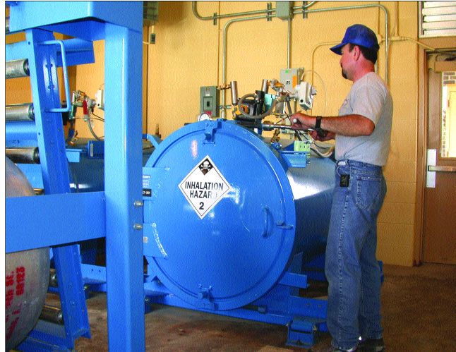
The photo above shows Leavenworth Water Department Operator Mike Domnick tightening bolts on the door of the containment vessel. Mike's comment is that this is the hardest part of the operation, by which he means the entire process is relatively easy.
