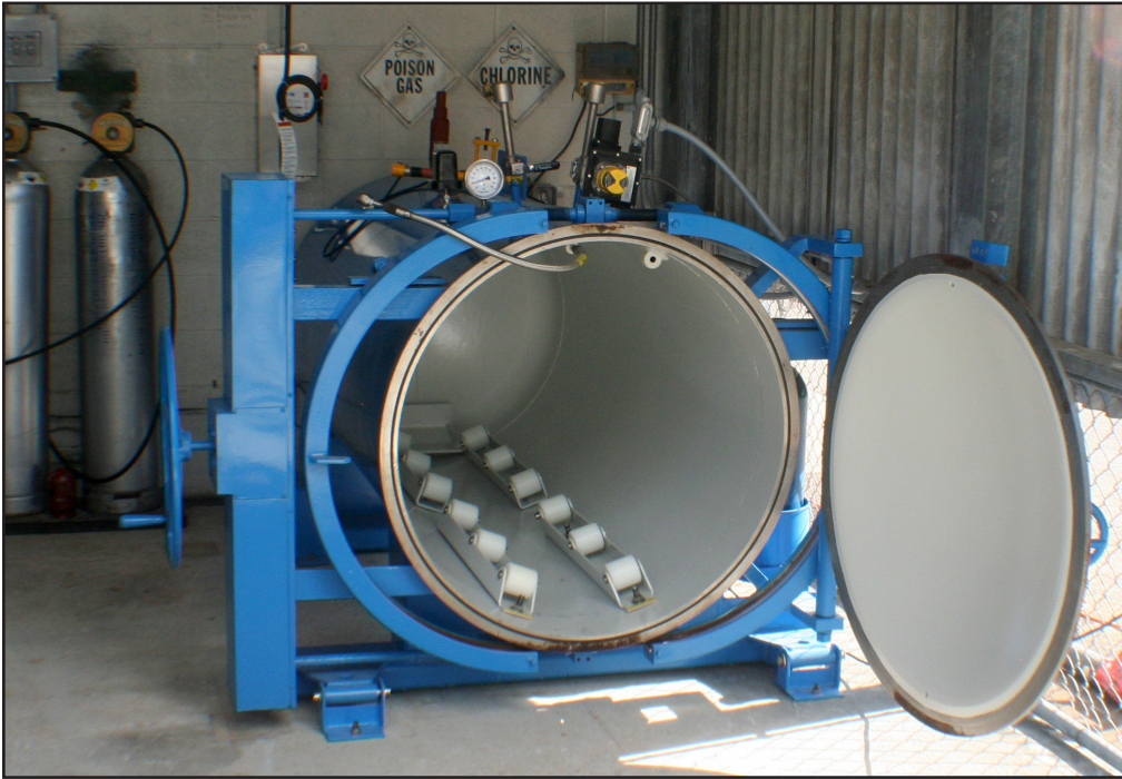
One-ton ChlorTainer™ cylinder containment vessels were supplied with loaders, scale systems, and instrumentation. Roller stands ease cylinder changing.
