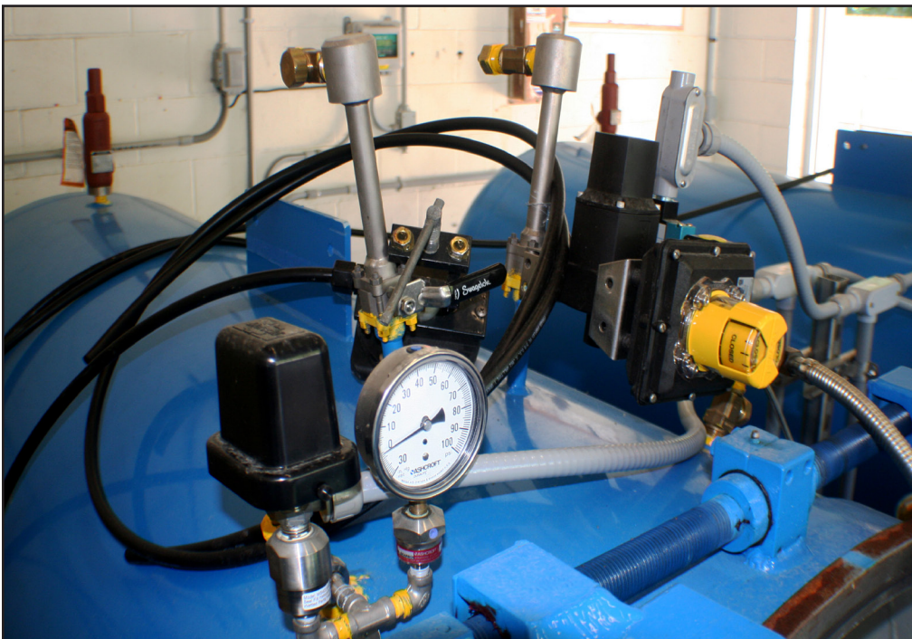
Instrumentation on top of units includes a failsafe valve that ties into the chlorine leak detection sensor, so that in the event of an external release, the failsafe valve will close, stopping any external leak.
