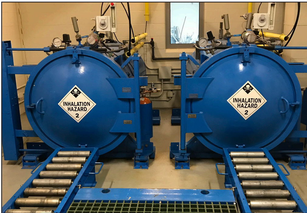
At the new plant, two 1-ton ChlorTainer™ cylinder containment vessels were supplied with loaders, scale systems, and instrumentation. Rollers ease cylinder changing.
