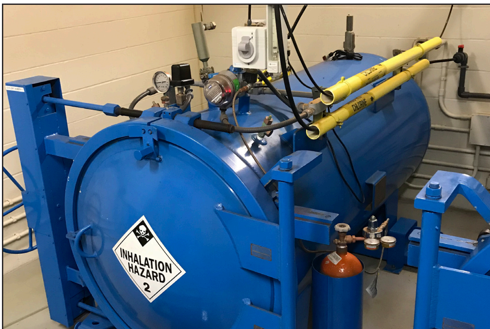
Instrumentation on top of the units include a failsafe valve that ties into the chlorine leak detection sensor, so that in the event of an external release, the failsafe valve will close, stopping any external leak.
