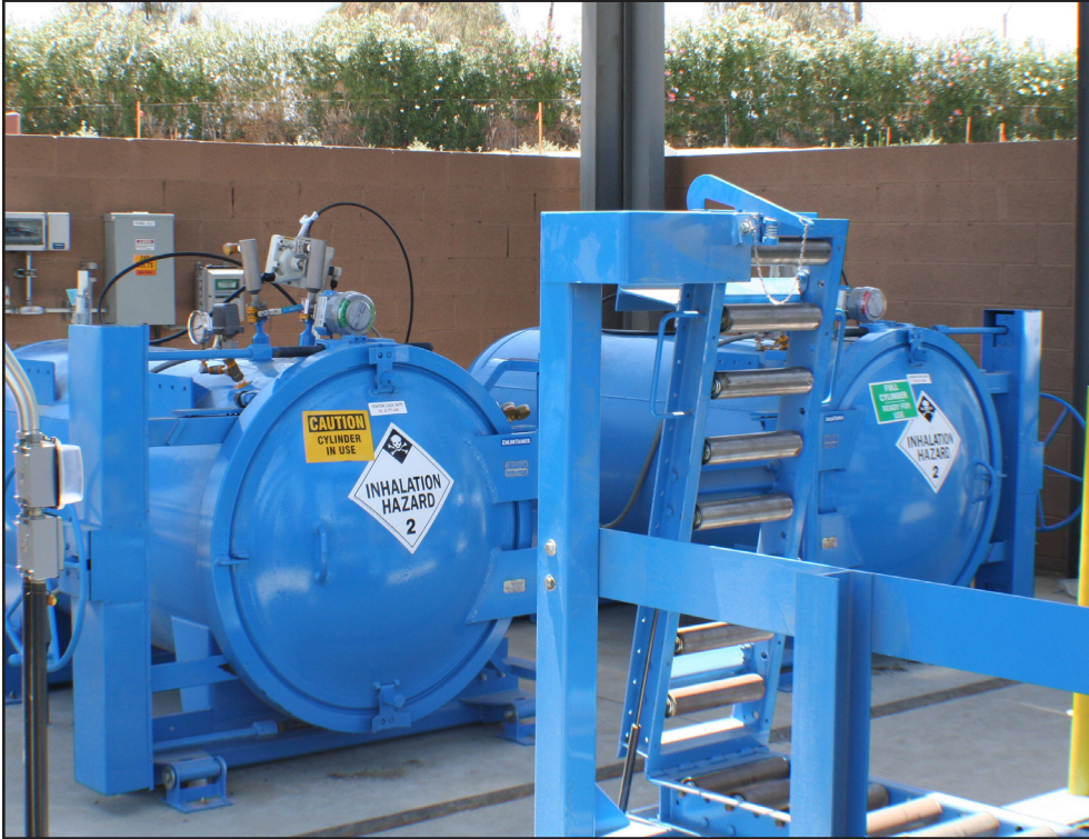
Two 1-ton ChlorTainer™ units like these, with one online and the other serving as a backup, are deployed at each of two arsenic treatment facilities (ATF's). When a cylinder switches over, a replacement is ordered for the empty. Any 1-ton cylinder with chlorine in it is always in a Chlortainer.
