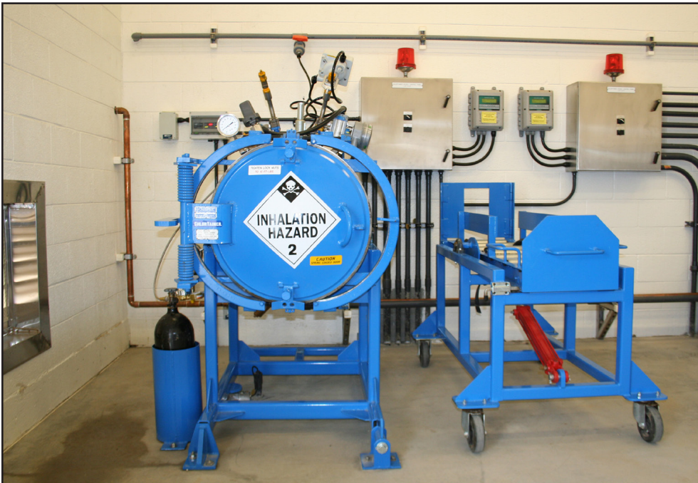
At the reservoir facilities, each has three 150-lb. ChlorTainer™ units like these. Each holds two cylinders, and both feed simultaneously. The three units are installed where chlorine-treated well water goes to the reservoir.
