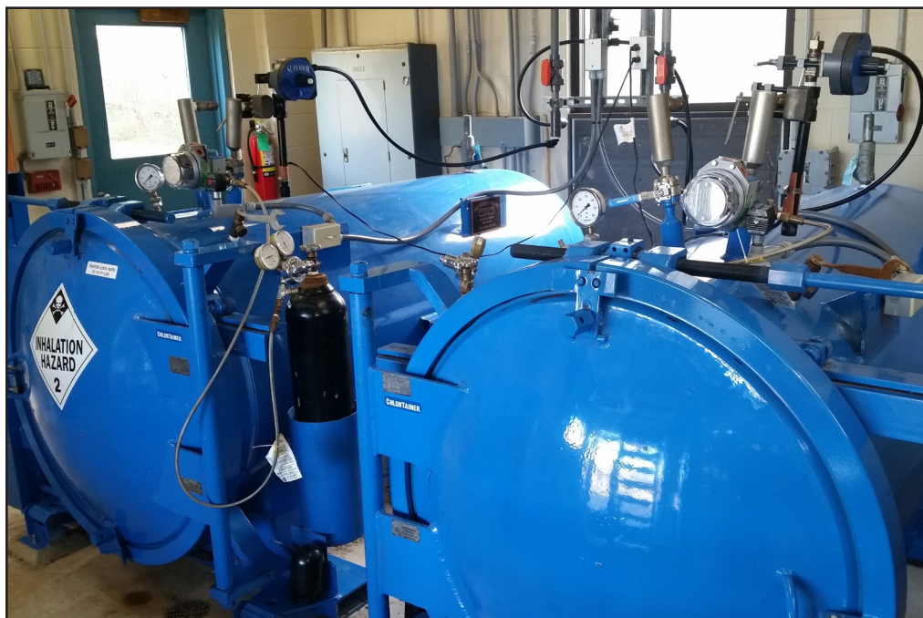
Containment vessels for sulfur dioxide cylinders, stored in a separate building, were similarly installed in 2012, with loader and scale system, and with fail-safe valves and vacuum regulators.
