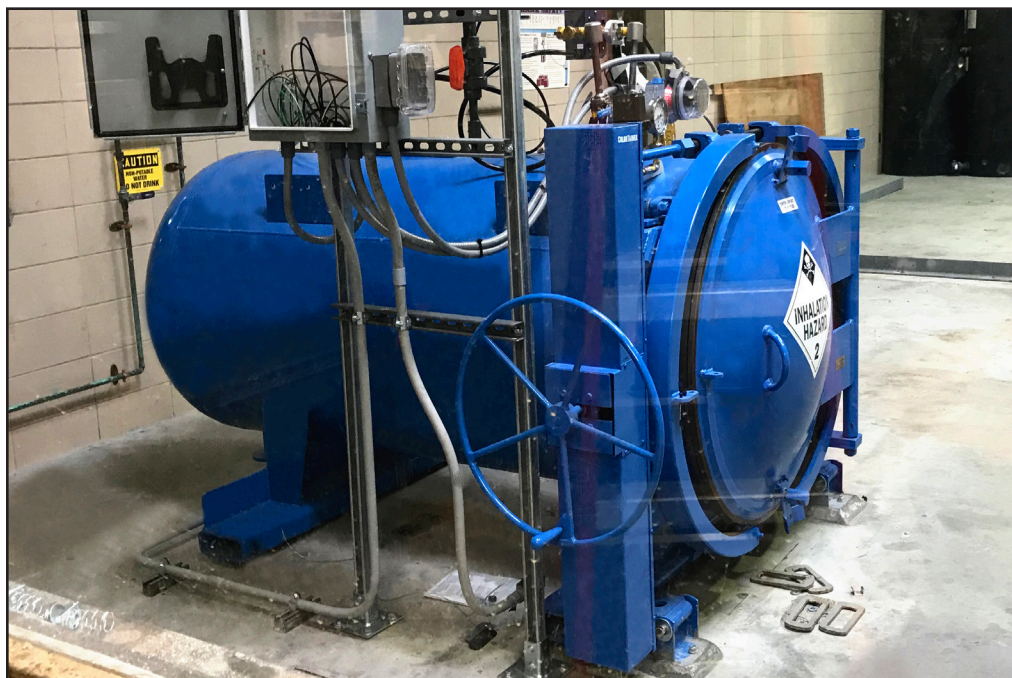
The one-ton ChlorTainer™ cylinder containment vessel was supplied with loader, scale system, and instrumentation. Roller stands ease cylinder changing.
