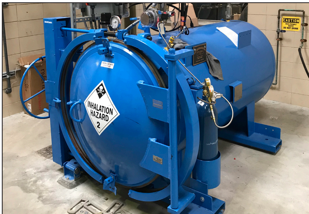
Instrumentation on top of unit includes a failsafe valve that ties into the chlorine leak detection sensor, so that in the event of an external release, the failsafe valve will close, stopping any external leak.
