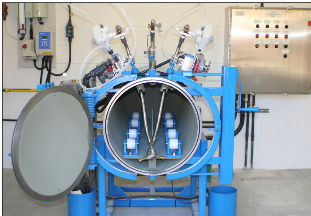
Two 1-ton cylinders of chlorine are stored in a covered building. The ChlorTainer™ containment vessels were installed in 2010 with a loader, scale system, and instrumentation also supplied. A failsafe valve ties into the chlorine sensor. A vacuum regulator can be attached to remove leaking chlorine inside the vessel.
