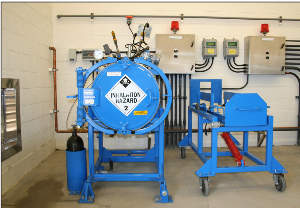
At the reservoir facilities, each has three 150-lb. ChlorTainer™ units like these. Each holds two cylinders, and both feed simultaneously. The three units are installed where chlorine-treated well water goes to the reservoir.
